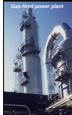
Gas-fired power plant
